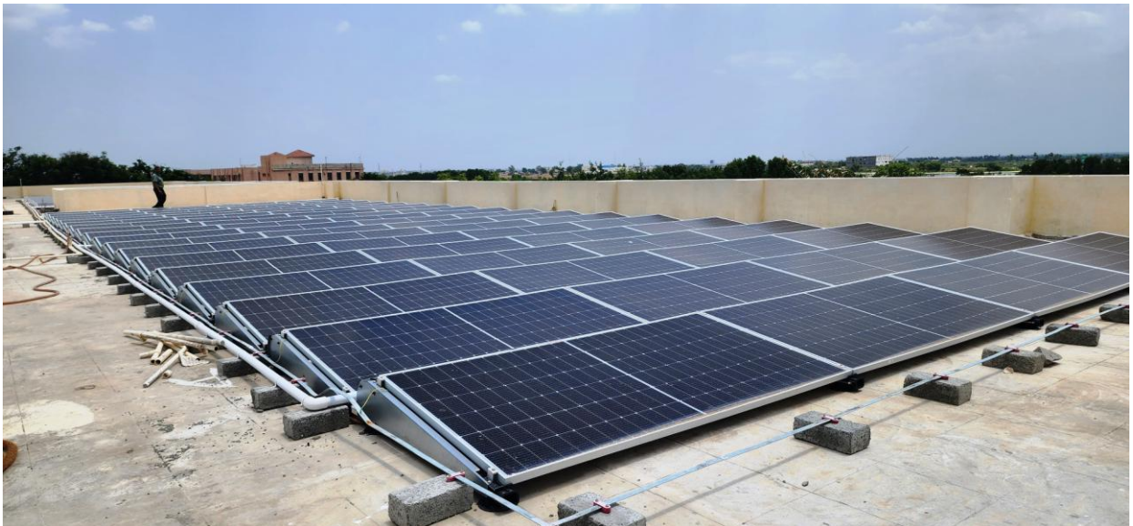
Solar Panels at VSU College
