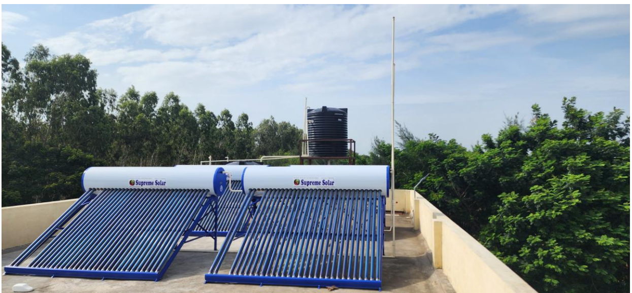
Women's Hostels Solar panels hot water tank
