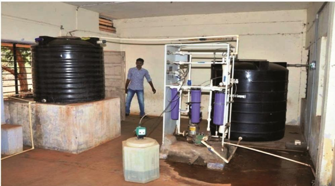
RO Water System
