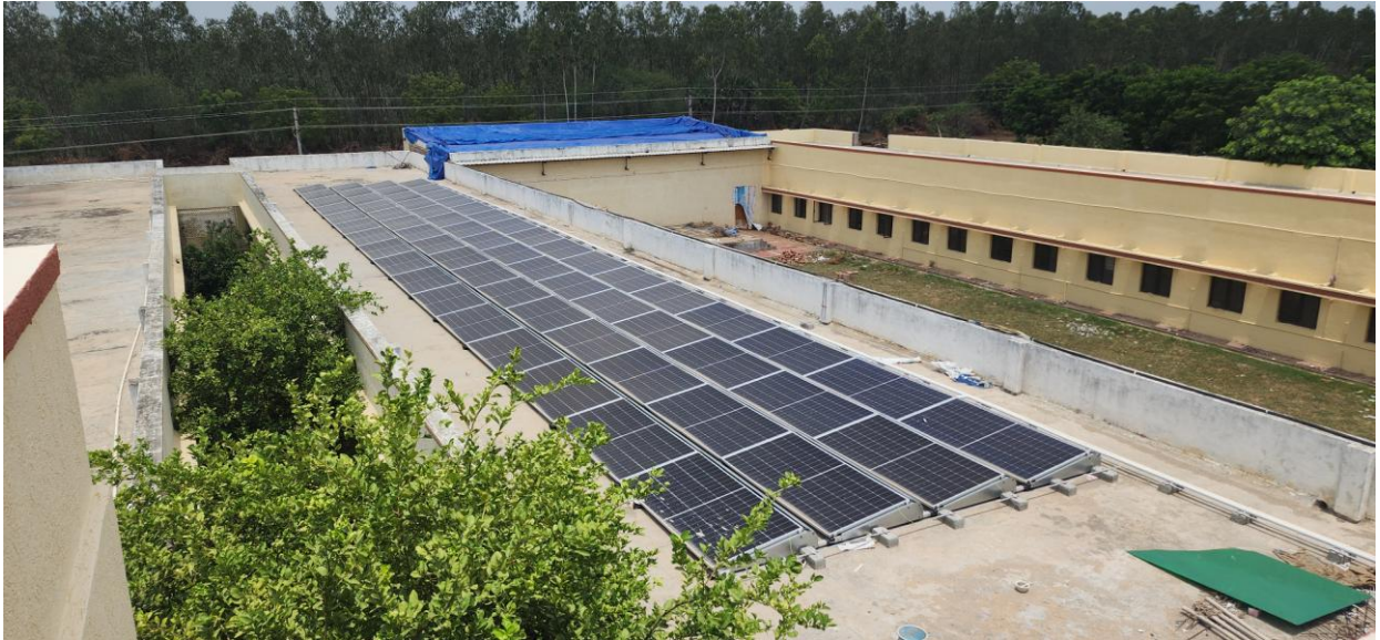
Solar Panels at VSU College
