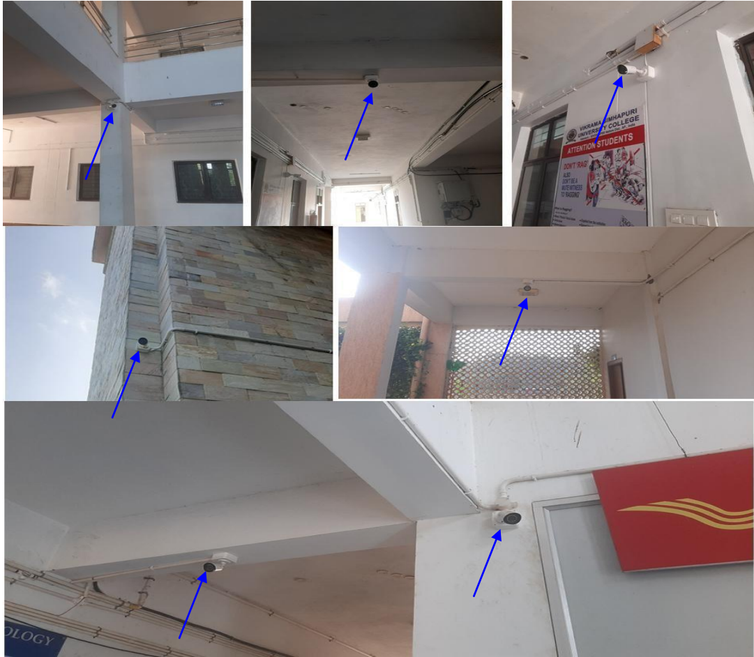
CCTV Camera's at SPSR Bhavan
