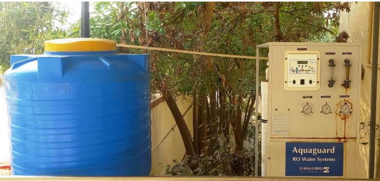
RO Water System
