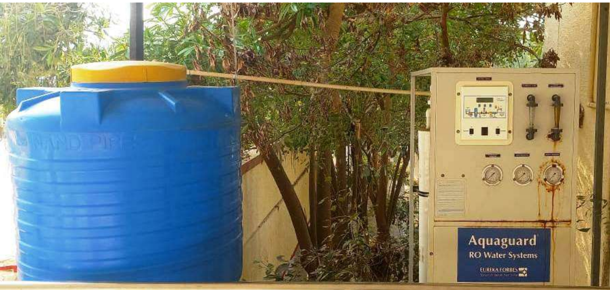
RO Water System
