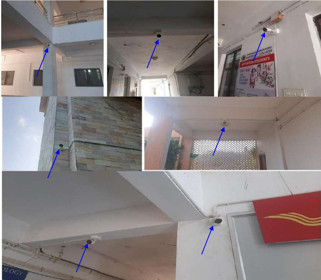
CCTV Camera's at SPSR Bhavan
