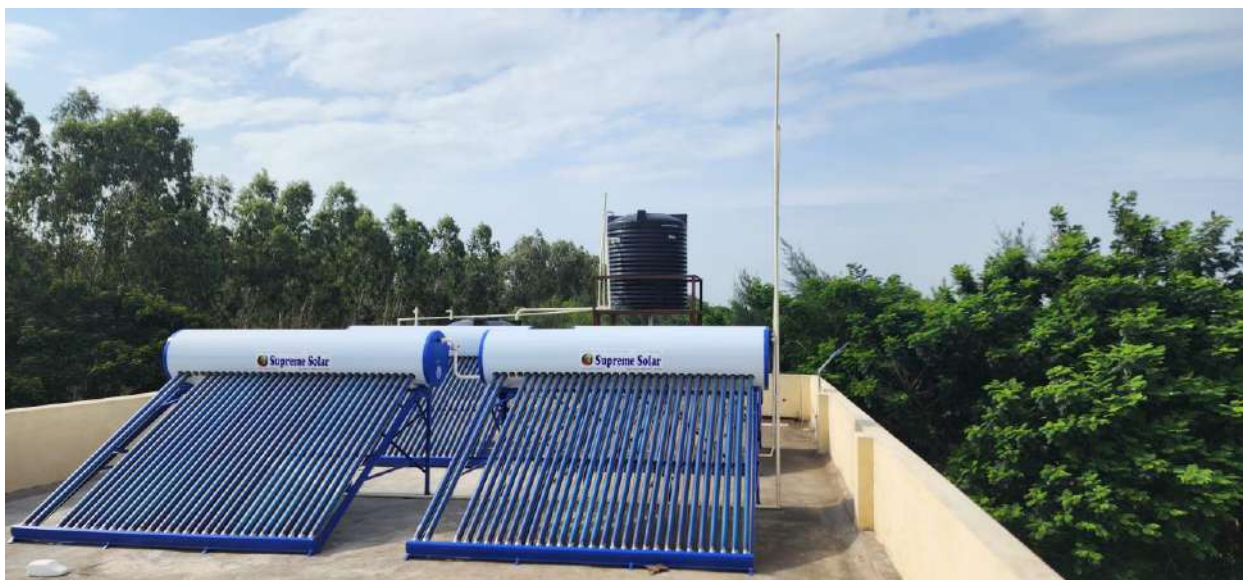
Women's Hostels Solar panels hot water tank
