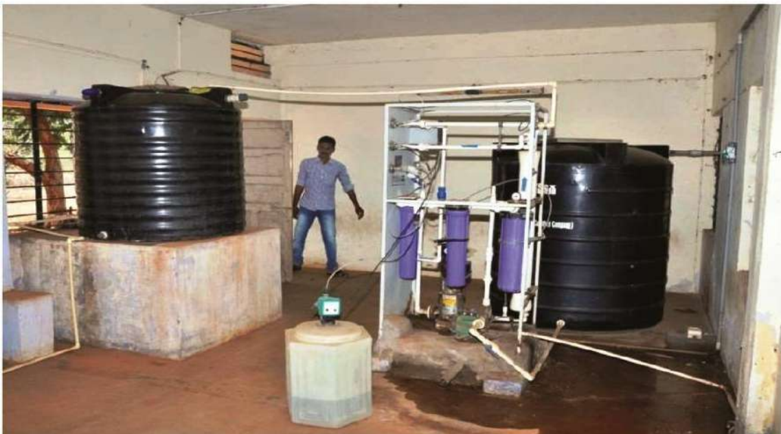
RO Water System
