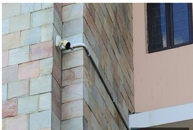
CCTV cameras at Administrative Building
