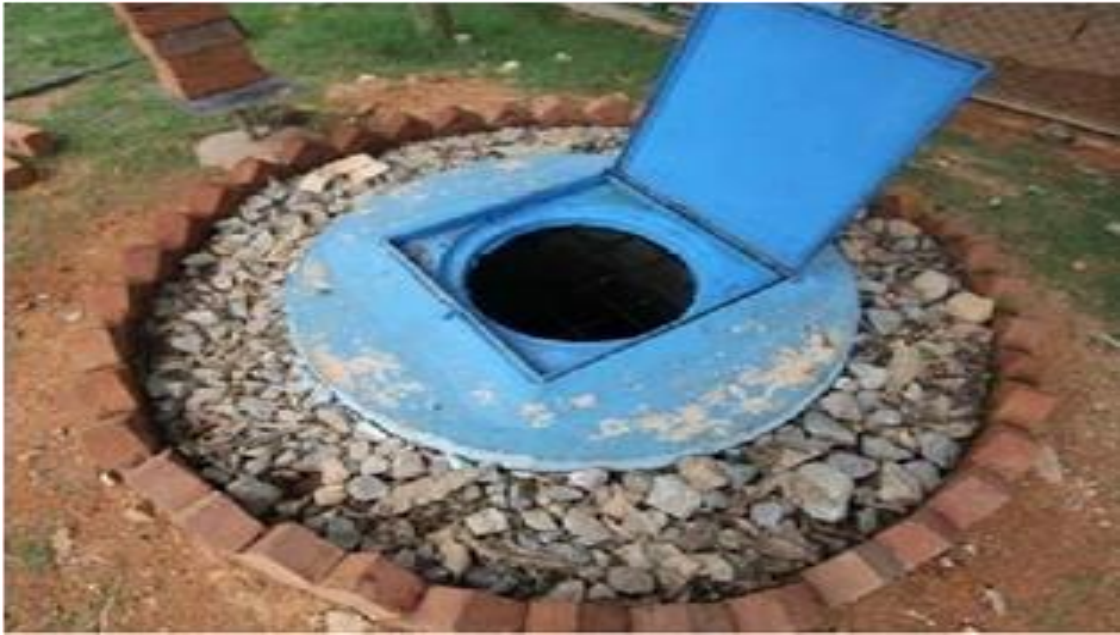
Roof top Rain water harvesting Pit
