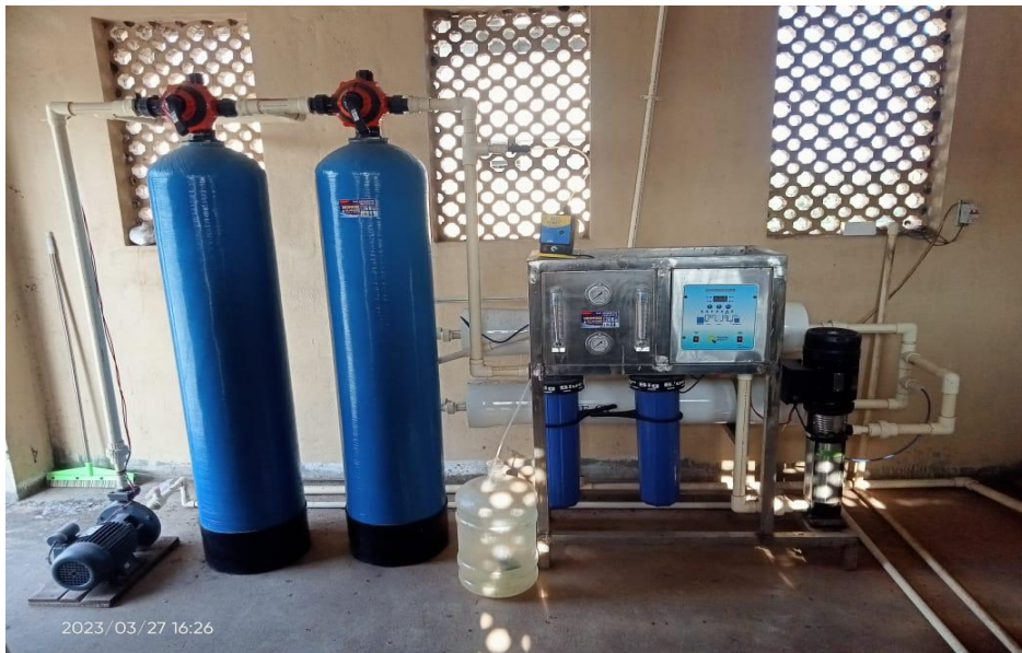
RO plant at VSU, Nellore campus
