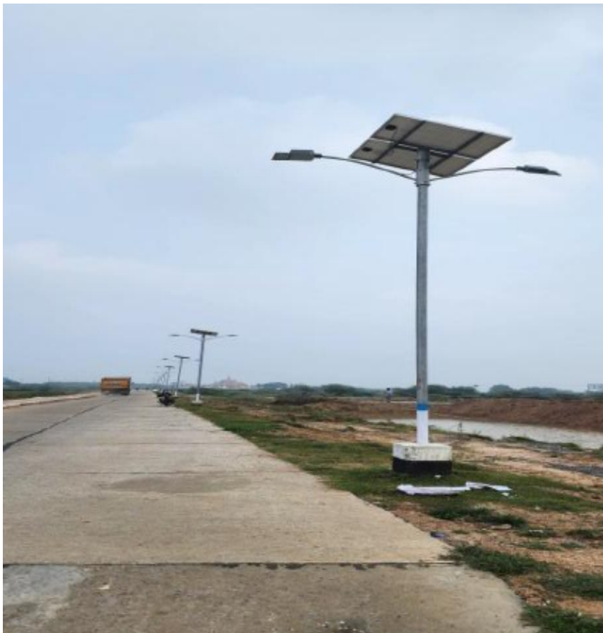
Solar panel LED lights in the common areas and roads in the campus
