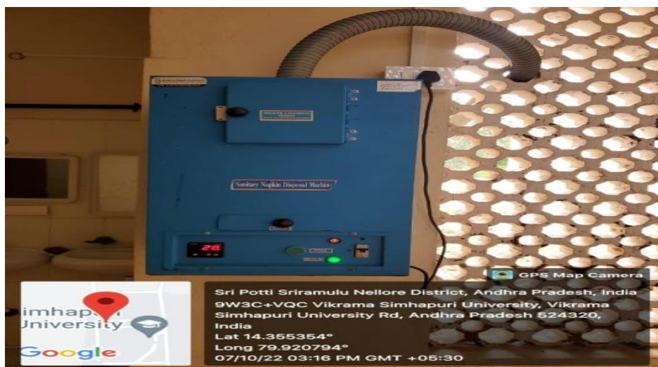
Sanitary napkin incinerator machine at Swarnamukhi women Hostel
