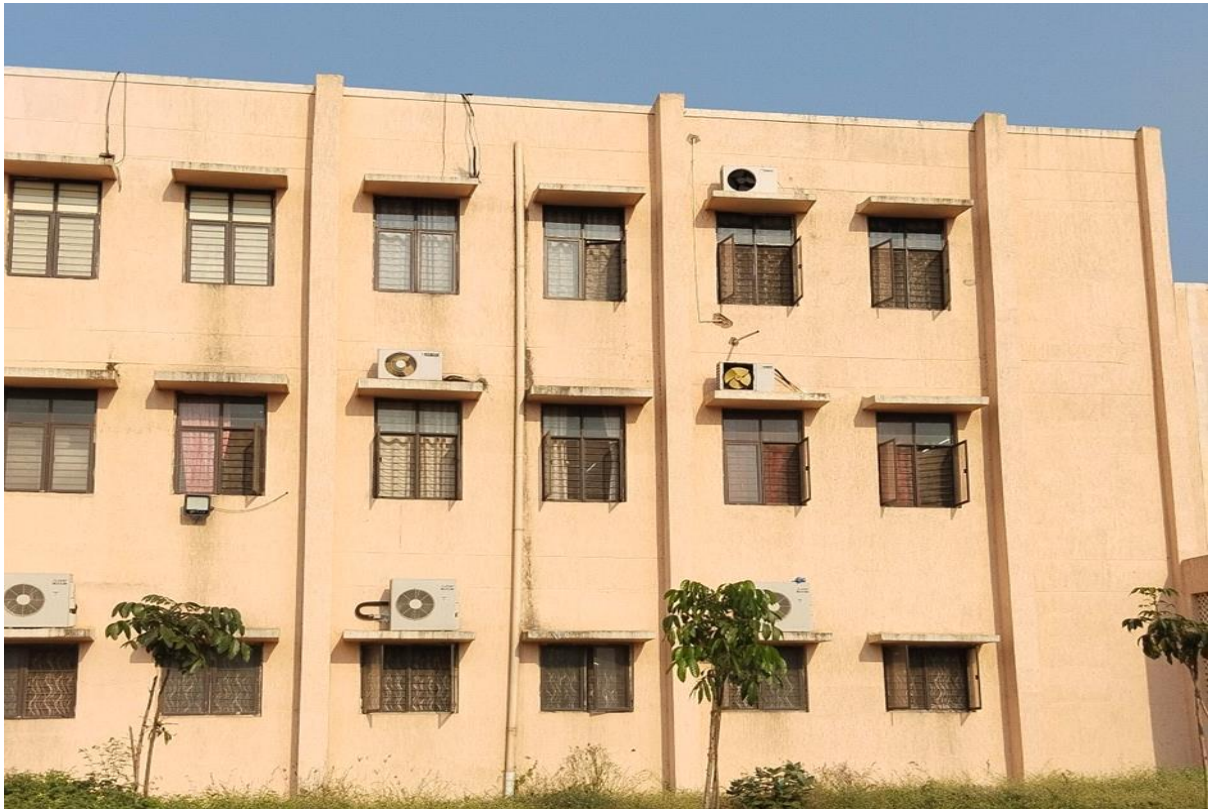
Roof top Rain water collecting pipes at AD building
