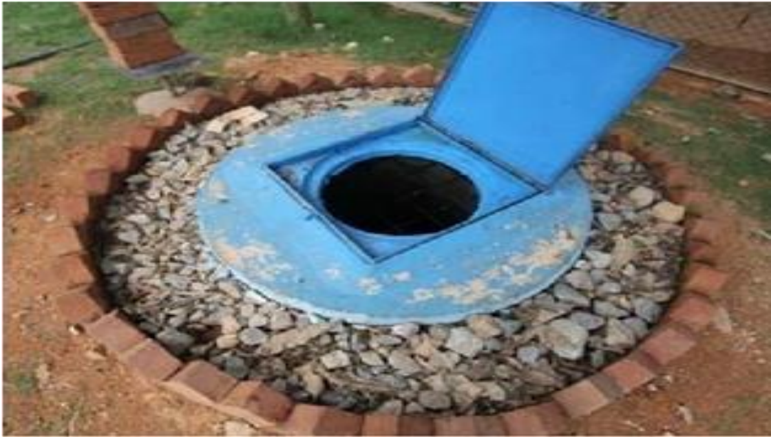
Roof top Rain water harvesting Pit
