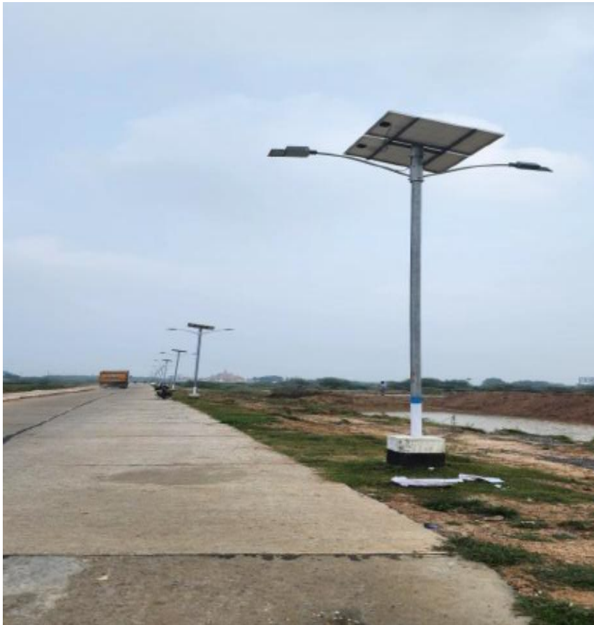
Solar panel LED lights in the common areas and roads in the campus
