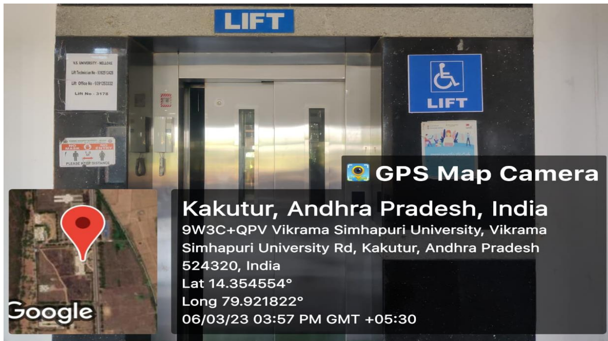
Lift facility with sign boards at AD Building
